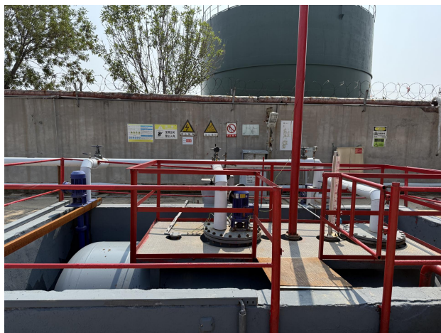
污水收集转运罐 ↑
